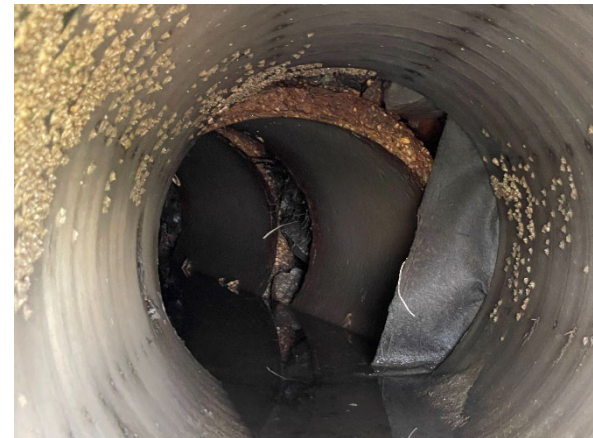
Outfall pipe Condition
