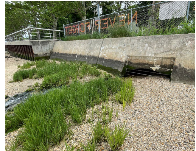
Outfall is over 50% filled
