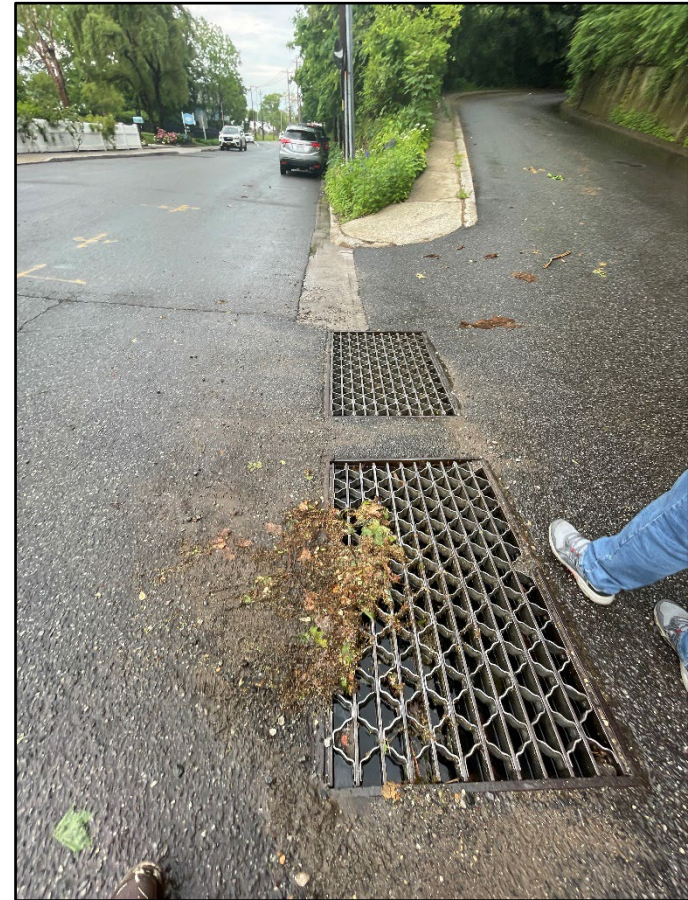
Structures do not connect to positive system
