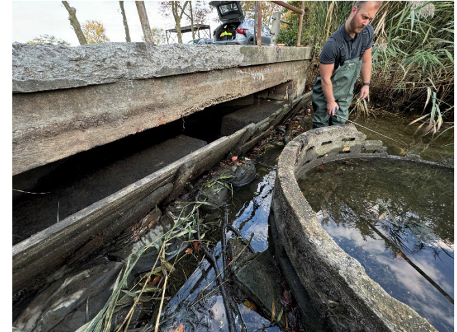
Timber Baffle Obstructing Weir
