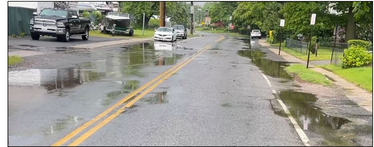
Poorly graded flow line
